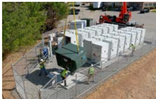
Battery storage in Pascoag
