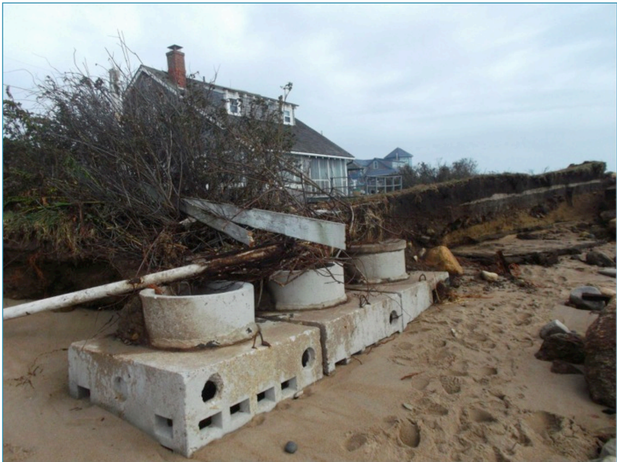
Exposed septic system: Erosion can uncover and damage septic systems during severe coastal storms.
