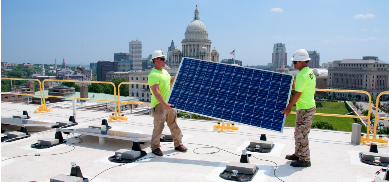
Solar array on the rooftop of Rhode Island's Department of Administration building.
